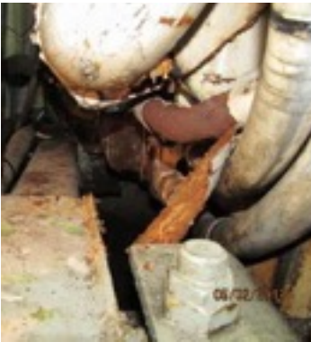
Outboard Port Engine (Rust and peeling paint)
