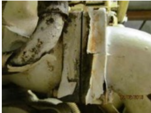
General Condition: Paint Peeling
