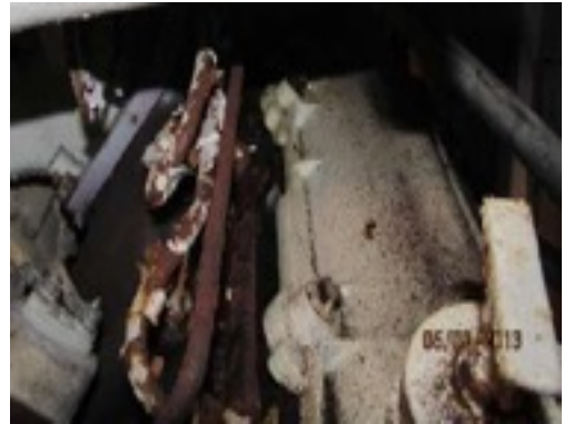
Rusted Fuel Lines
